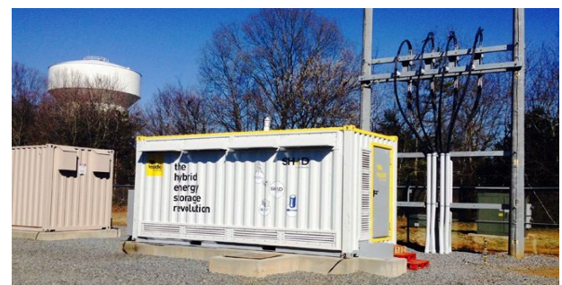
Figure 4: Hybrid energy storage system at Duke Energy [24]
