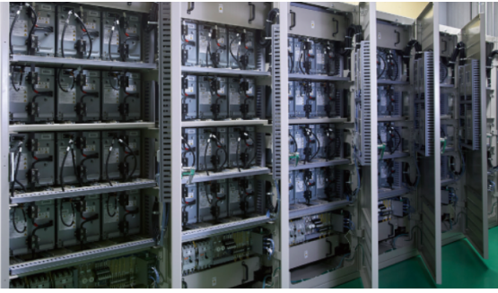
Figure 5: (a) Supercapacitor banks [25]
