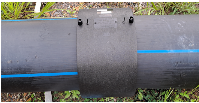
Figure 12: A HDPE pipe joint
