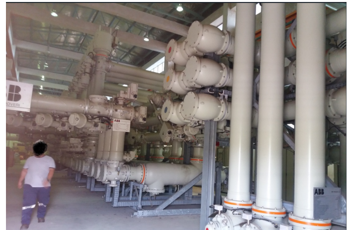
Figure 4: GIS substation in Bintulu, Malaysia which uses GIL lines.
